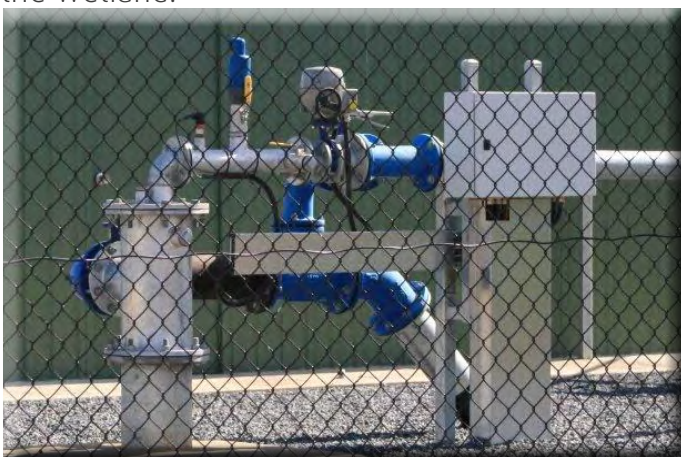
Injection headworks at Greenfields
