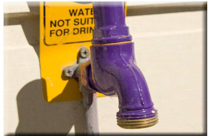
Purple tap used to supply recycled water
