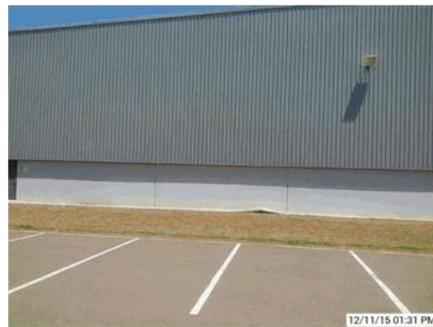
Rear of Warehouse Including Pedestrian Walkway – Note Lifted Concrete Pathway
