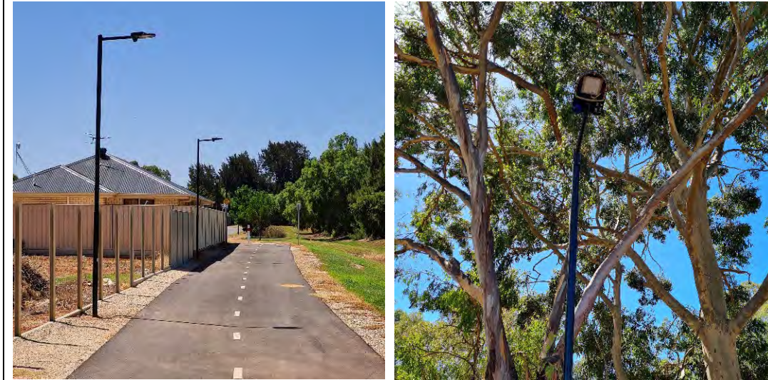
Gawler Greenway, Parafield Gardens, Trail Lighting
