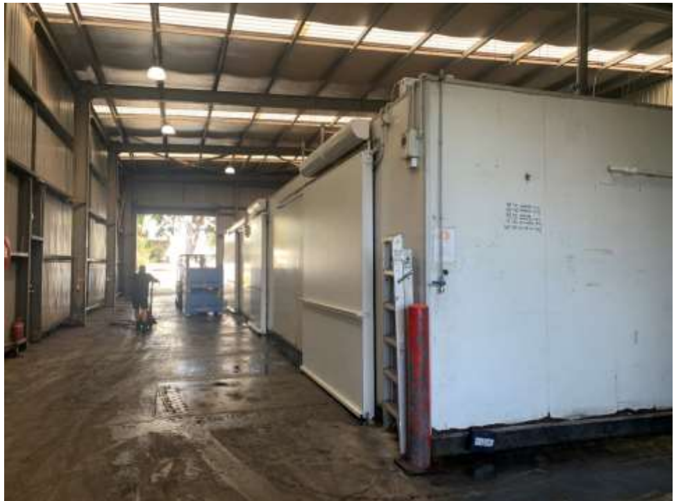
Photo 4. Internal arrangements – existing coolrooms.
