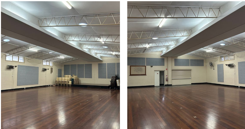
Acoustic Panels at Pooraka Farm Memorial Hall
