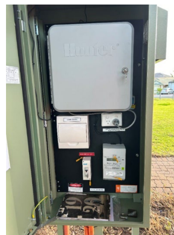
New Irrigation Controller Cabinet at Springbank Waters
