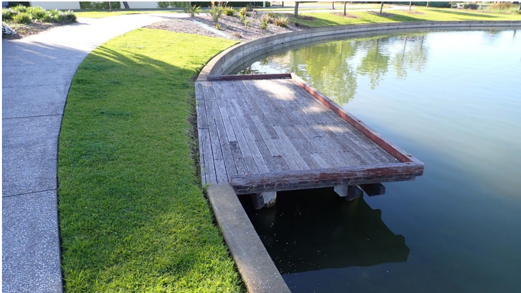
Example - Viewing/Water Activity Deck/Wharf Structure, BRIDGE-178 Nelson Crescent Lake Reserve, The Bridges Village, Mawson Lakes
