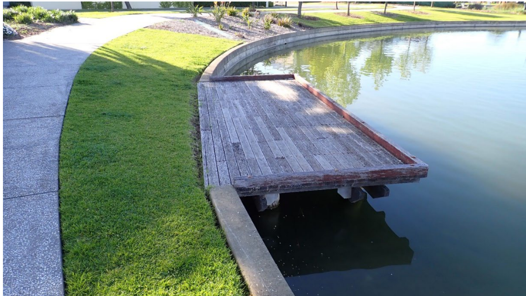
Example - Viewing/Water Activity Deck/Wharf Structure, BRIDGE-178 Nelson Crescent Lake Reserve, The Bridges Village, Mawson Lakes
